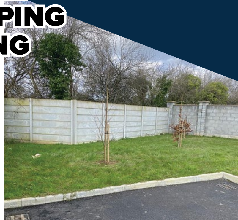
This is a photo of an item on a snag list from a builder. Kerry County Council wants the builder to remove the fence and replace it with a fence that's a few inches taller. Because there is a slope in the green area the fence measures 2 mtrs when measured from the back and 1.85mtrs when measured from the front because of the slope in the green area. Does it really matter if this fence is a few inches shorter. This is an example of the nonsense that builders have to put up with from Kerry County Council.
