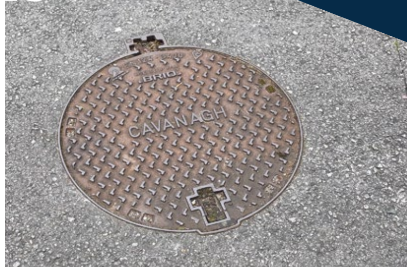
This is a photo of a manhole that was built in 2008. This manhole is in perfect condition after sixteen years.
