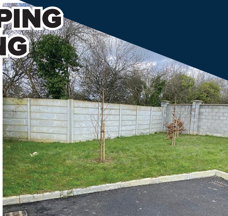
This is a photo of an item on a snag list from a builder. Kerry County Council wants the builder to remove the fence and replace it with a fence that's a few inches taller. Because there is a slope in the green area the fence measures 2mtrs when measured from the back and 1.85mtrs when measured from the front because of the slope in the green area. Does it really matter if this fence is a few inches shorter. This is an example of the nonsense that builders have to put up with from Kerry County Council.
