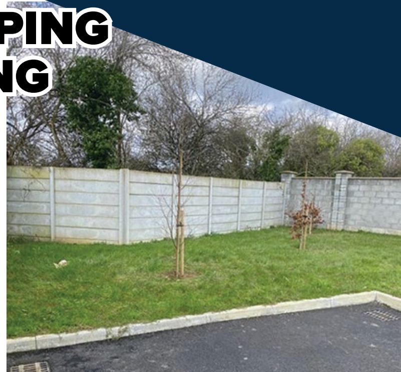
This is a photo of an item on a snag list from a builder. Kerry County Council wants the builder to remove the fence and replace it with a fence that's a few inches taller. Because there is a slope in the green area the fence measures 2 mtrs when measured from the back and 1.85mtrs when measured from the front because of the slope in the green area. Does it really matter if this fence is a few inches shorter. This is an example of the nonsense that builders have to put up with from Kerry County Council.
