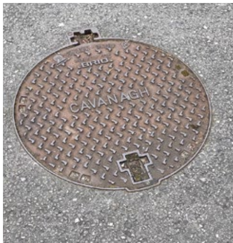
This is a photo of a manhole that was built in 2008. This manhole is in perfect condition after sixteen years. The specifications on building a manhole has changed recently and Kerry County Council wants all the manholes in the estate dug up and rebuild under the updated specifications and this work will cost the builder €45,000. Kerry County Council does not accept that this decision is a gross abuse of power. There is no appeal system and no consequence for the decision makers.
