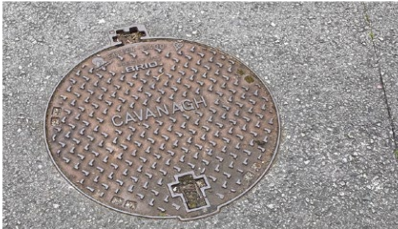
This is a photo of a manhole that was built in 2008. This manhole is in perfect condition after sixteen years.
