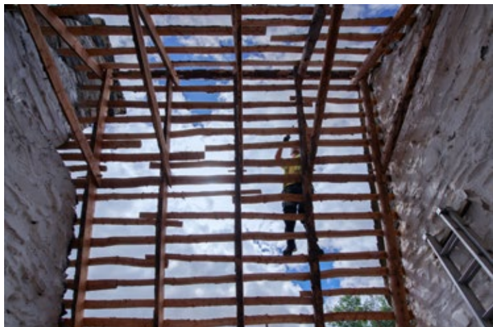
Traditional Thatcher, Lukasz Shalec working on the roof of Foley's Farmhouse Project - using traditional material, The project is funded by the Trustees of Muckross House and Gardens, for the reroof, rethatch and provision for under floor geothermal heating system. The aim is to preserve the fabric of the building for future generations - the project using master craftsmen should last 200 years. Photo: Valerie O'Sullivan
