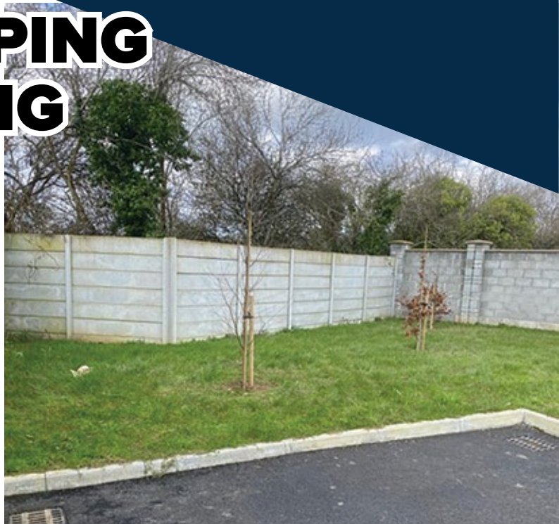
This is a photo of an item on a snag list from a builder. Kerry County Council wants the builder to remove the fence and replace it with a fence that's a few inches taller. Because there is a slope in the green area the fence measures 2 mtrs when measured from the back and 1.85mtrs when measured from the front because of the slope in the green area. Does it really matter if this fence is a few inches shorter. This is an example of the nonsense that builders have to put up with from Kerry County Council.
